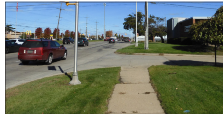
Sidewalk gaps, utility pole locations conflict with potential sidewalks along some segments.
